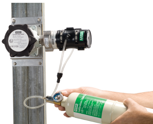
Figure 11 Bump Check setup with environmental guard
